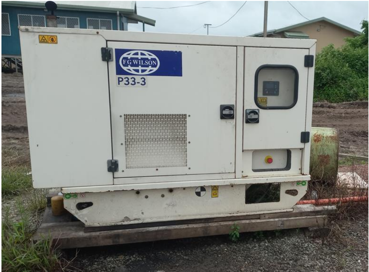
Figure 22. Existing Temporary 33 kVA FG Wilson Generator
