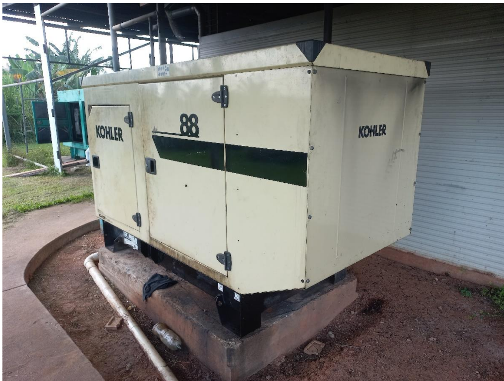
Figure 10. Top: Existing 80 kVA Kohler generator. Bottom: Nameplate of existing 80 kVA Kohler generator
