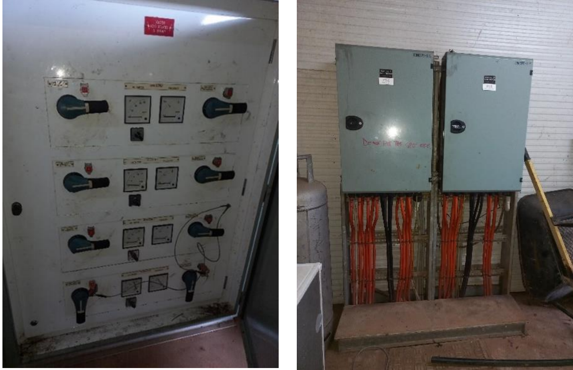
Figure 9. Left: Existing switchgear – manual changeover switches for four sources. Right: Hospital essential and non-essential mains distribution board
