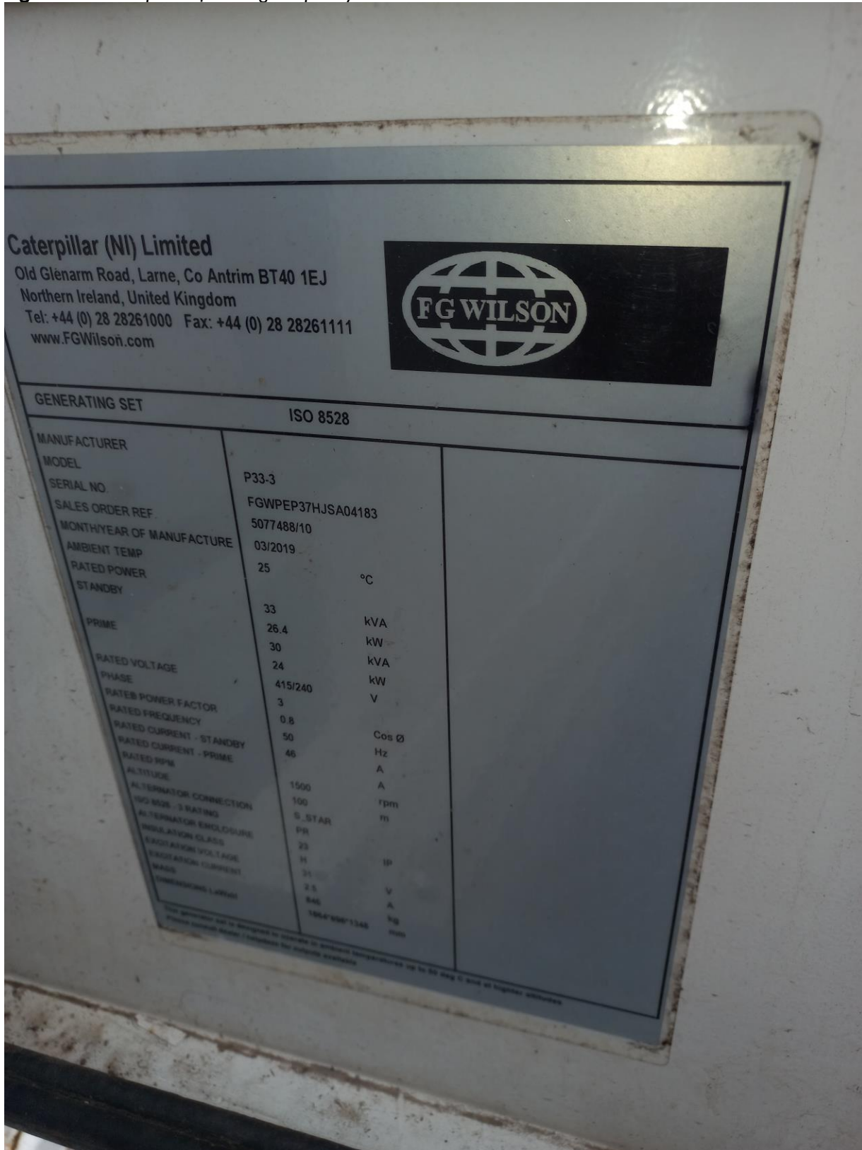
Figure 23. Nameplate of existing temporary 33 kVA FG Wilson Generator
