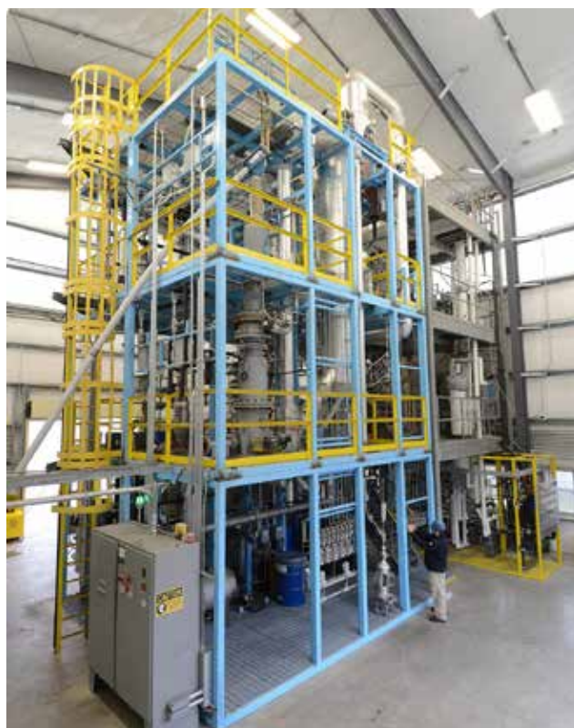
RTI 1-ton-per-day catalytic biomass pyrolysis pilot unit
