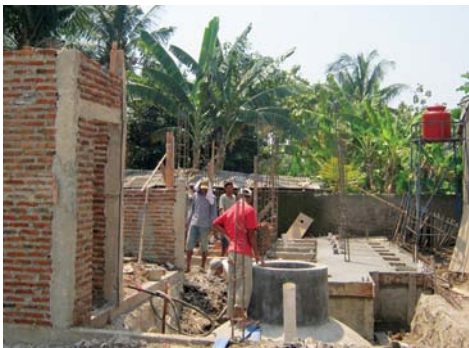
RTI trains local masons to build tanks used for the on-site wastewater treatment provided for toilet blocks.
