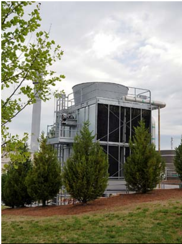
The cooling towers are part of the chilled water production system at the central utility plant on RTI's main campus.
